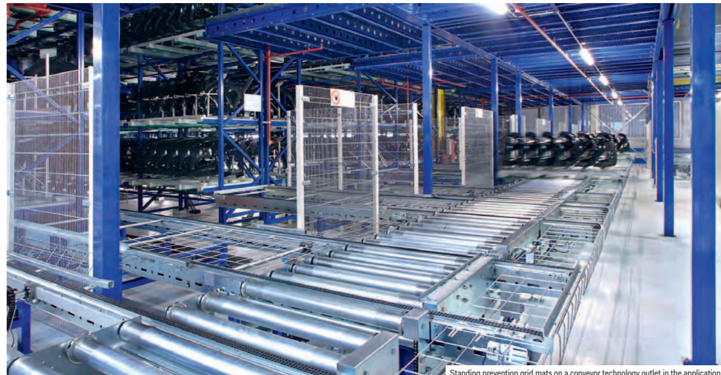
Standing prevention grid mats on a conveyor technology outlet in the application
